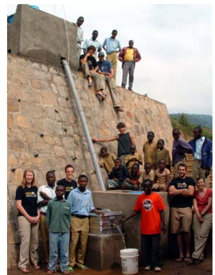
EWB-CU Rwanda team members in front of newly installed BYOW system
